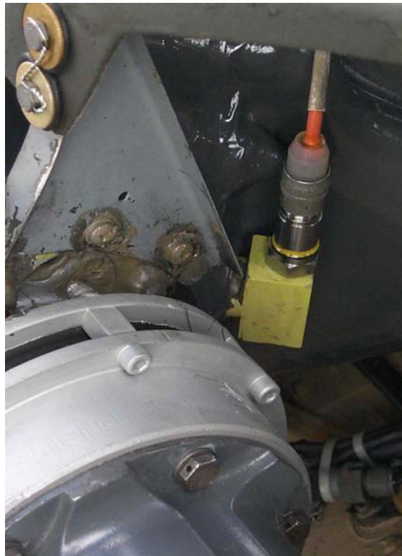
Figure 19. No. 1 Input Module Accelerometer Installation (ACC1)
