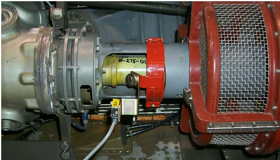
Figure 24. No. 1 Engine Output Shaft Optical Tachometer Sensor Installation
